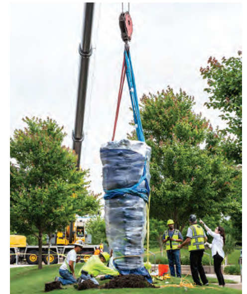
Workers use a crane to lift Dumna and place it on Seldin Plaza.
