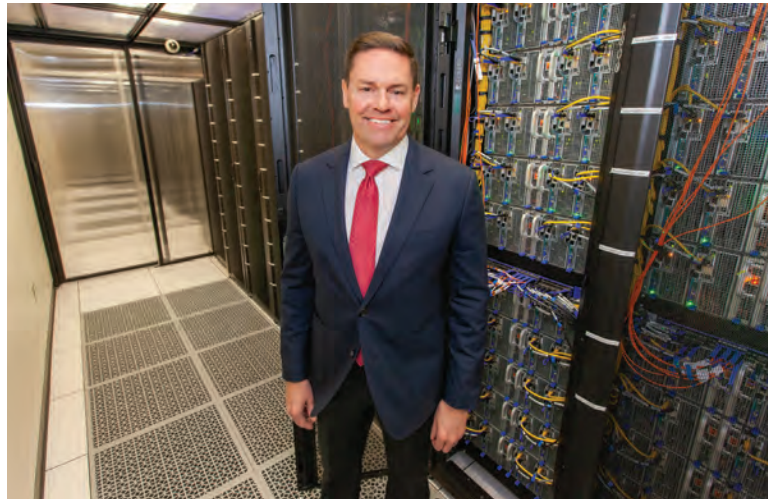
Byron Davis in UT Southwestern's data center
