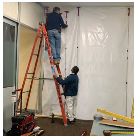
Painter Americo Alvarez and carpenter Victor Israelian work on a containment barrier at the newly renovated clinic inside the Bass Center.
